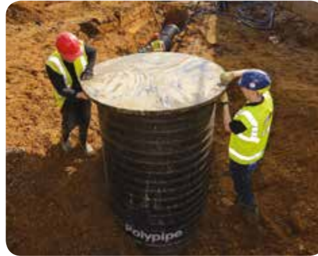
Polypipe delivers a unique earth tube project as part of the redevelopment of Westbrook Primary School
