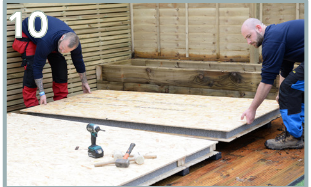
Place the fourth floor panel (F), knock into the third panel and ensure it sits flush on the final floor bearer. Repeat the process using 35mm screws between the third and fourth panels.
