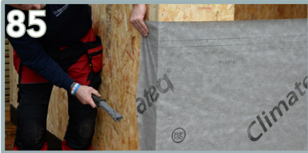
85 Then wrap the excess around the corner and staple the starting point into place.
