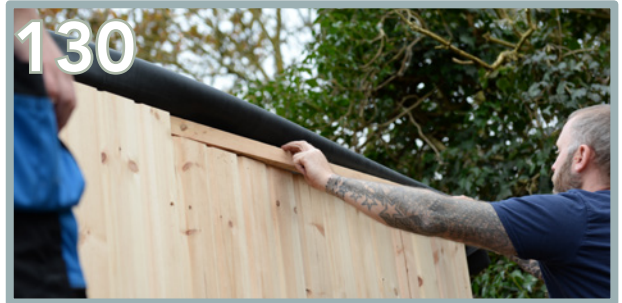
To install the Angled Roof Battens, lift the EPDM and slot the matching batten's listed in the components list into place above each T&G Side Panel (BB, BH & BA).
