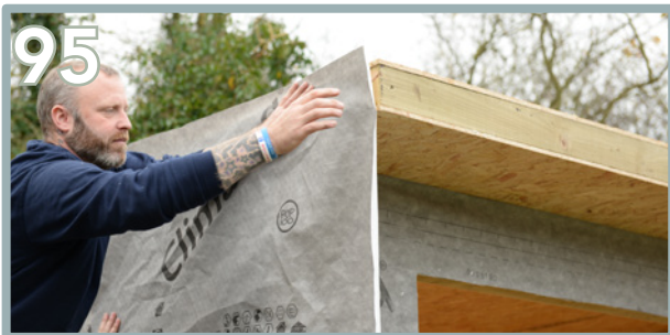
Use the excess membrane to cover the angle on the side panels and roof overhang.
