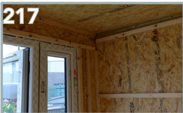
217 Use 5 x 80mm screws for each batten. The battens on the left hand side will not be aligned to the front batten positions.
