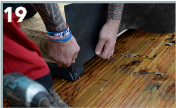
Start to unwrap the DPC roll and choose a starting point on the base's outer face. Ensure it covers half of the bearers and staple into place.
