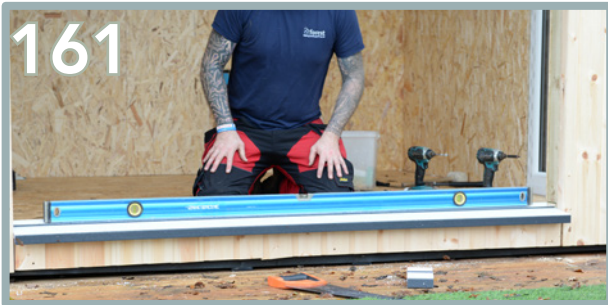
Place the ledge onto the silicone. Ensure it is level and the back edge meets the first edge of the back OSB sheet (the same positioning as the window).
