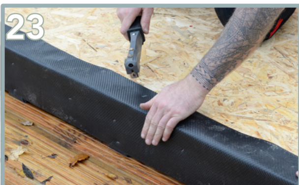
Continue folding the overhang and corners of DPC onto the OSB sheets as you make your way around and staple into place.
