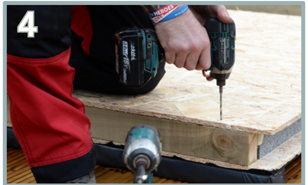
4 Pre-drill for every process before securing with screws. Pre-drill 5 holes along the edge of the first floor panel. Do not screw in the other side at the moment.
