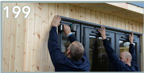
199 Position the top plastic 'L' strip across the door. Pre-drill the face underneath and fix first.
