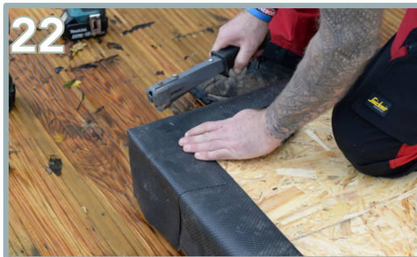
Using a Stanley knife, cut the DPC at the corner to create 2 pieces to easily fold onto the OSB sheets and staple into place.
