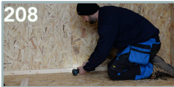
Repeat the process at the bottom of the wall, ensuring the second batten is flush with the floor and end to end. Use 5 x 80mm screws along the batten at equal spaces.
