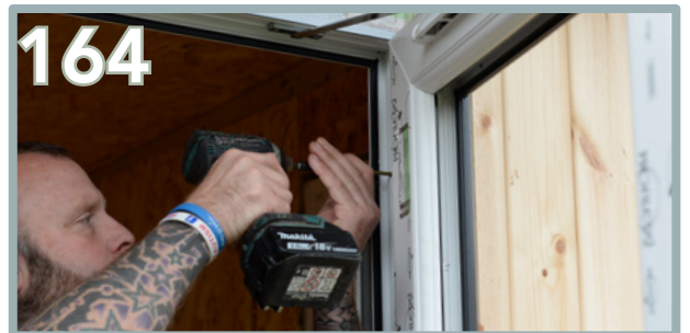
These should be drilled 150mm from the top and bottom corners and 300mm from the 150mm points with the 112mm/100mm screws.
