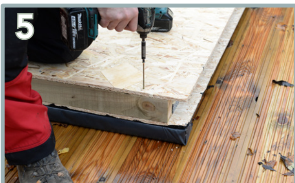
5 Using 125mm screws, screw through the floor panel into the floor bearer beneath. Repeat the process for the 4 other screws. Ensure each screw is countersunk.
