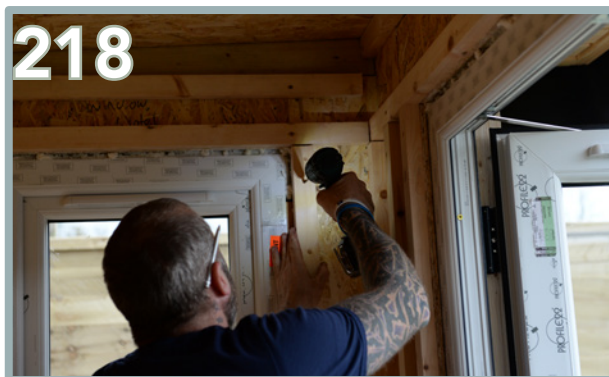
218 On the right-hand wall, secure a batten at the top of the wall, in line with the top back wall batten, using 5 x 80mm screws. Secure a second batten along the wall so it is flush with the top of the window frame. Finish framing the window by securing a 45x28x1960mm batten on either side of the window using 4 x 80mm screws for each batten.
