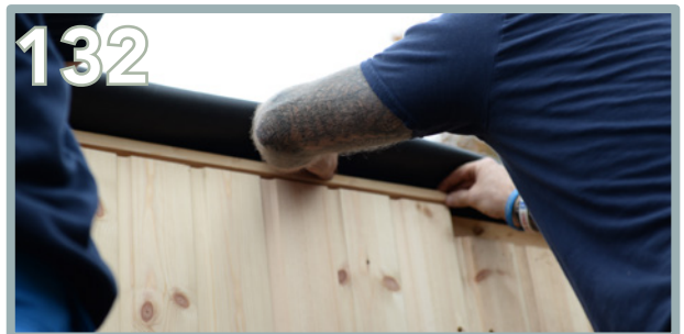
Repeat the same process for the other batten's on top of the other T&G Side Panels (BB, BH & BC). Screw into place using 2 x 80mm screws. Repeat the process on the opposite side.
