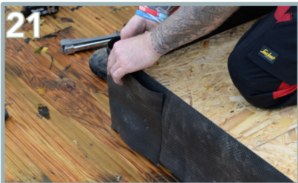
Once fully wrapped around the base, overlap the starting point and staple into place.
