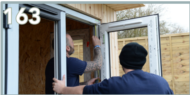
Check the frame is both level and plumb, then drill fixing holes into the frame side.
