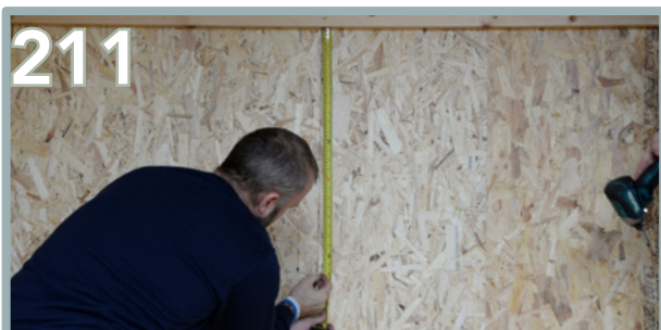
Repeat the same process to measure and mark out the position for the fourth back batten.
