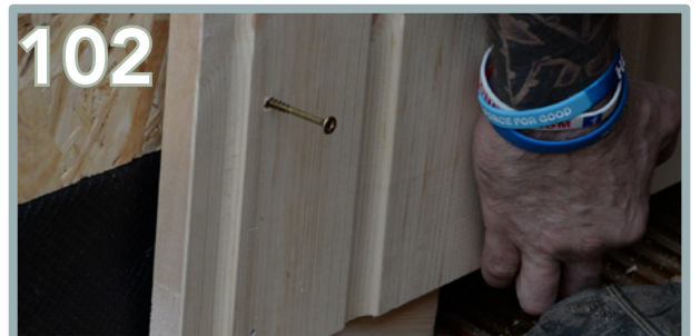
Use 6 x 80mm screws to secure each cladded panel (3 screws down each side). Screw through the batten on the panel and into the wall behind. Leave the screws slightly out in case of adjustment.
