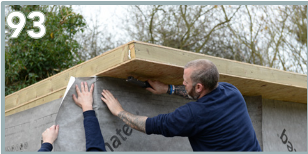
Using the excess membrane, cover the front flush up to the roof.
