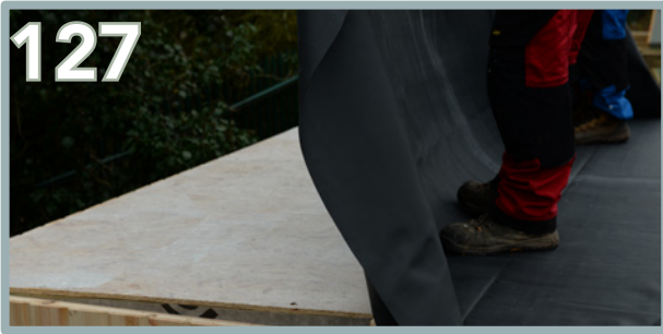
Apply glue to this side of the roof, making sure to reach all edges.
