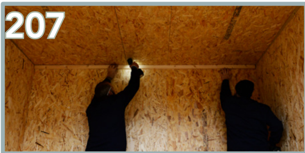
Begin at the back and position the first 45 x 28mm batten flush to the top. This will be the correct length to fit in the space end to end. Use 5 x 80mm screws along the batten.
