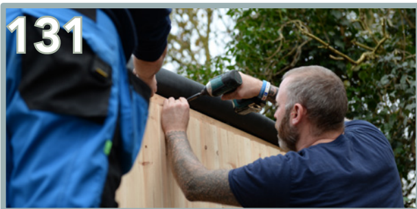
Screw into place using 2 x 80mm screws. Ensure the batten is butted up to the T&G panel and wall panel behind.
