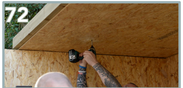
Pre-drill and screw 5 x 35mm screws, where the adjoining panels intersect. This will secure the roof panels together. Then secure the first roof panel's corners with 2 x 150mm screws.
