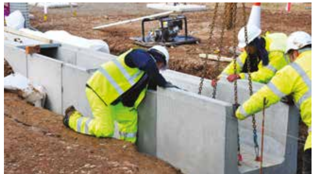
4. Lift slowly and with care, then place trough in position. Ensure trough is in line and level. Then remove lift chains and unscrew lifting loops.
