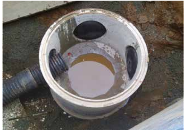
Can be used in straight through, 90° connection or straight through with a cross drain.
